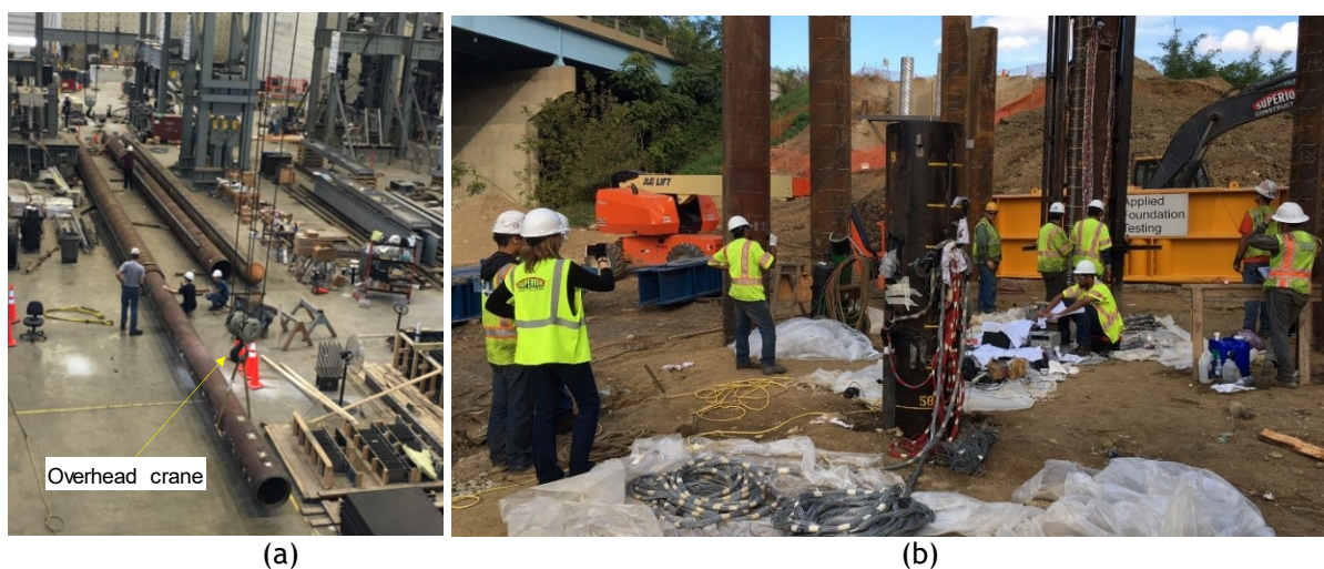
Figure 9. Static and dynamic load tests on large-diameter open-ended pipe pile: (a) assembly of the double-wall system; (b) on-site operations at the end of pile installation;
